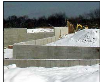
Proper stabilization prior to the onset of winter helps avoid issues during spring snowmelt.
